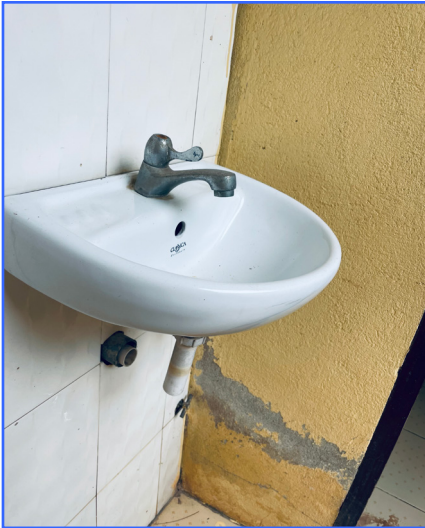
Broken sinks in Ghana.
